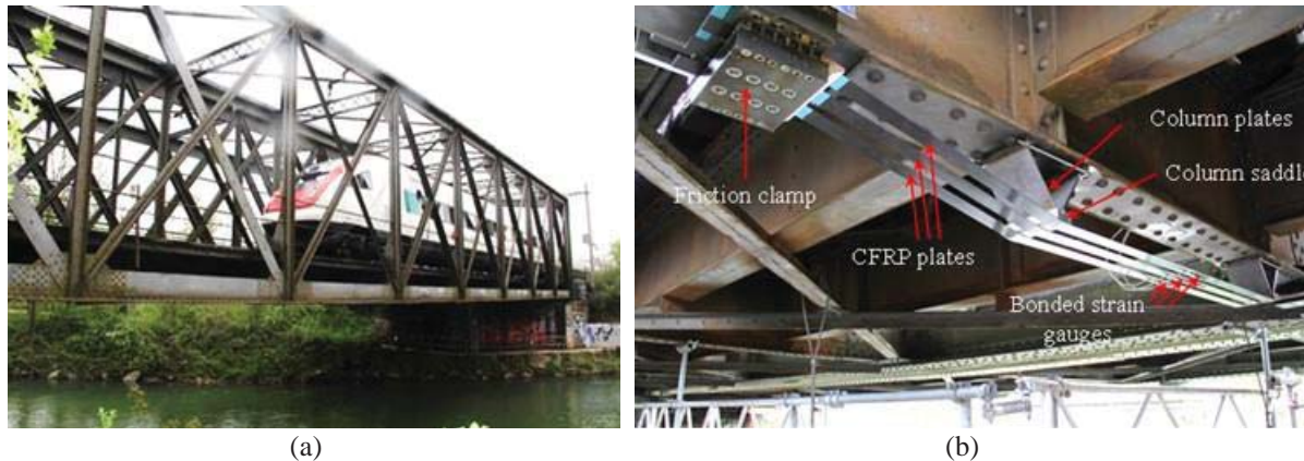
Figure 6. (a) Münchenstein railway metallic Bridge (120-year-old) subjected to a passenger train. The bridge consists of 10 panels with the total length of 45.2 m, width of 5 m and height of 6.15 m and built on a 45-deg skew. (b) The cross-girders were retrofitted with pre-stressed un-bonded CFRP strips (Ghafoori et al. 2015b).
